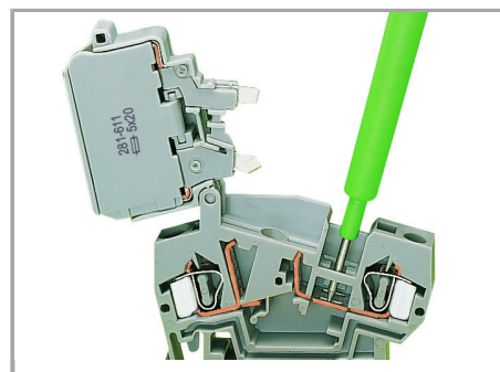
Voltage test at input in the test slot of the current bar
