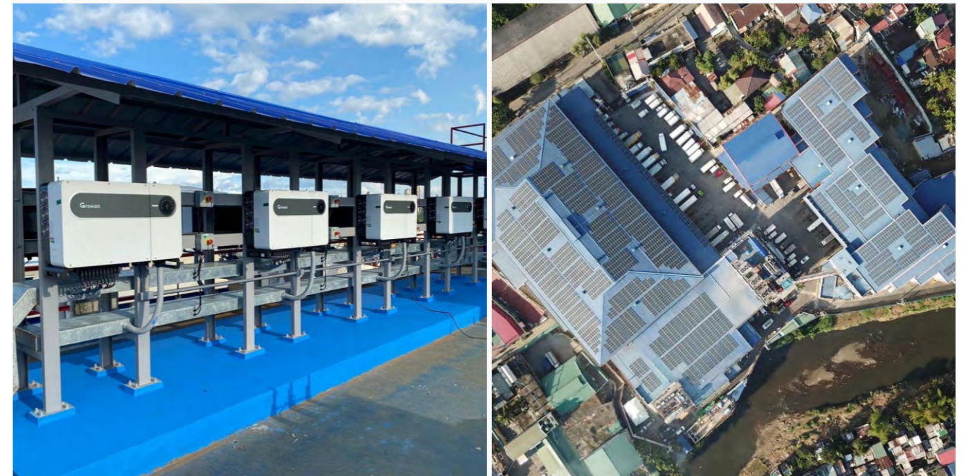
CASE STUDY: Philippines with 1.2MW solar installation.
