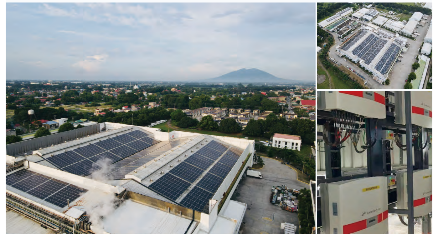
CASE STUDY: Pampanga, Philippines 1.3MW.
