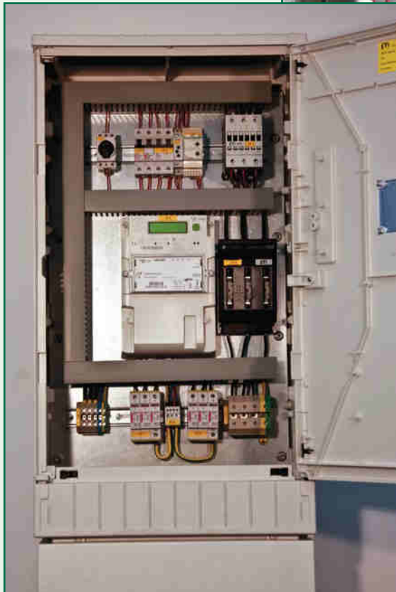
Meter distribution cabinet
