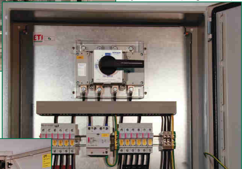
DC junction box (CH gPV fuses)
